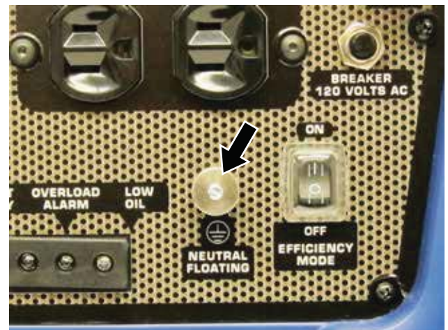
Figure 9 – Ground Terminal on the Control Panel
